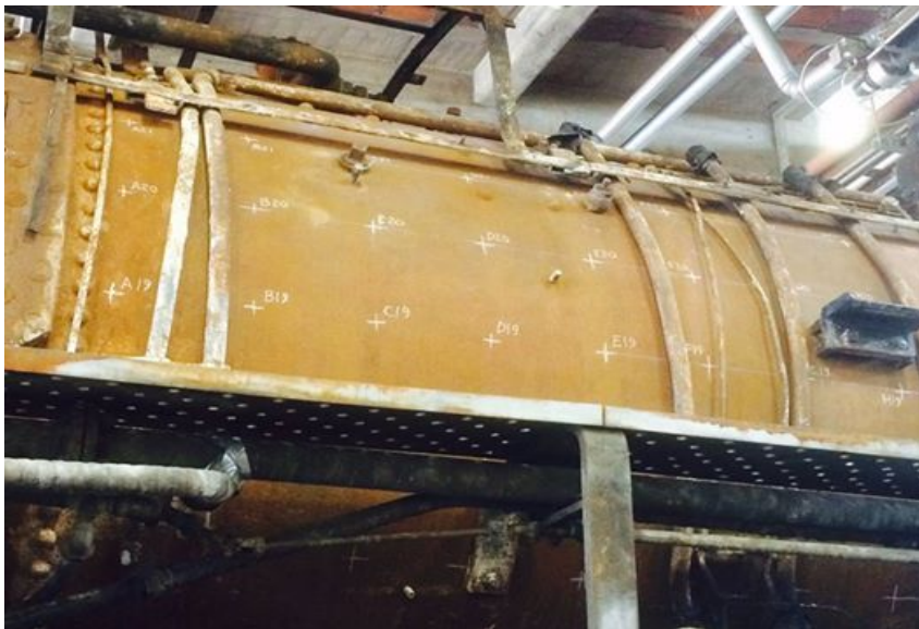
Gridlines on the boiler guide the ultrasound. Photo by Scott Lindsay.
