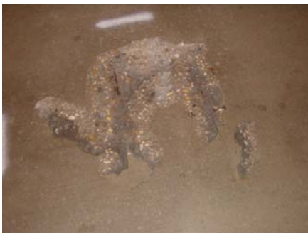
(Left: Exposed rebar in cement floor at Stamford station)
