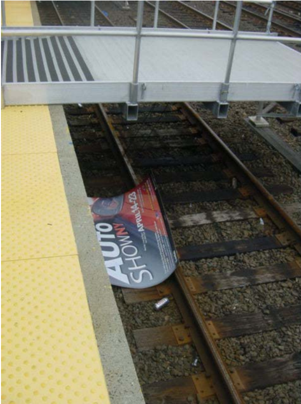
Trash on the tracks under bridge plates.
