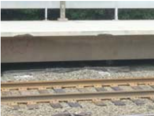
Platform crumbling from beneath.
