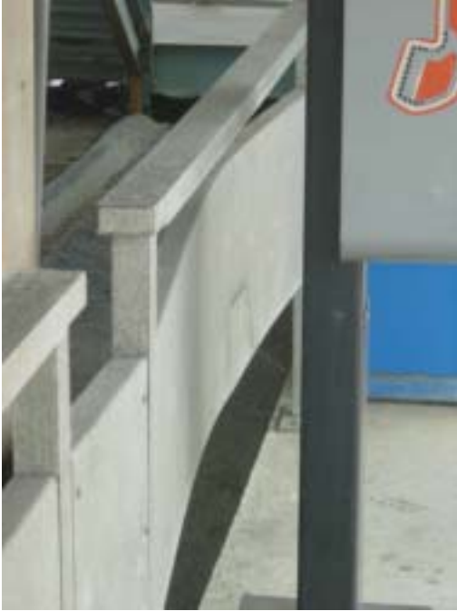
Platform siding bowed outward.
