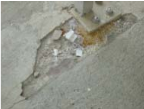
More “divots” in the concrete.
