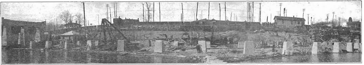
Panorama of Sunnyside Crossing Showing Abutment and Footings for Steel Trestle Approach.
