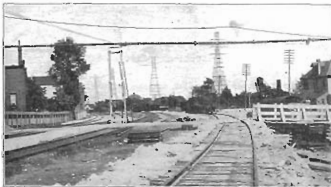
Looking East at Dunn Street While the First Shovel Cut Was Being Made.
