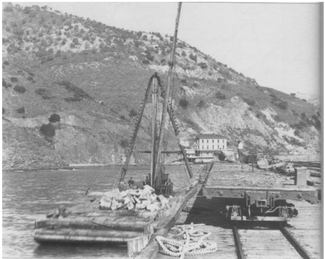
Figure 1: Transfer of Bishop Peak rock from flat car to barge for the Avila breakwater sometime between 1898 and 1905. The chains visible adjacent to the coupler were used to haul the flatcar up the incline to the Bishop Peak Quarry. Credit: San Luis Obispo County Historical Society as published on page 34 in The Pacific Coast Railway: Central California's Premier Narrow Gauge by Westcott and Johnson.
