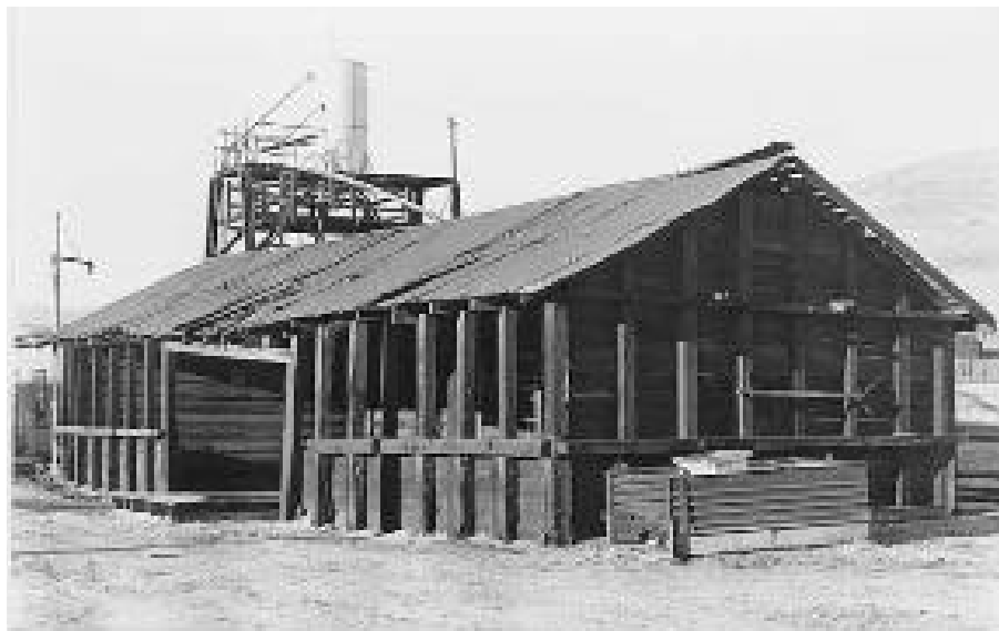
Figure 2: The sand house from the southeast side showing the condition in the early 1970 when maintenance was not existent. The photo does show the numerous bolted on supplements to the original columns which have dry rotted out at their base. Photo: Andrew Merriam, 1972
